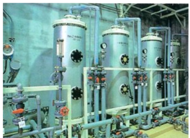
Filtration and Adhesion Tower
