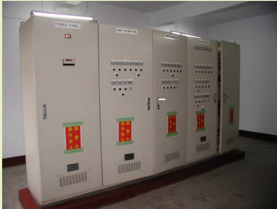
Main Control room
