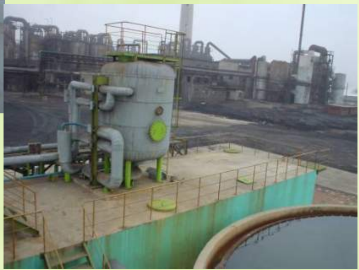
Sand filtration treatment
