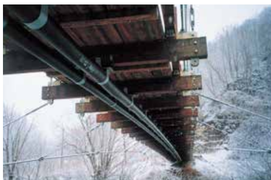
●橋梁添架配管●
